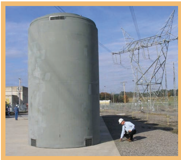
Scott Atwater, Region IV DNMS inspector, checking dry fuel storage casks at Arkansas Nuclear One in Russellville, AK.
