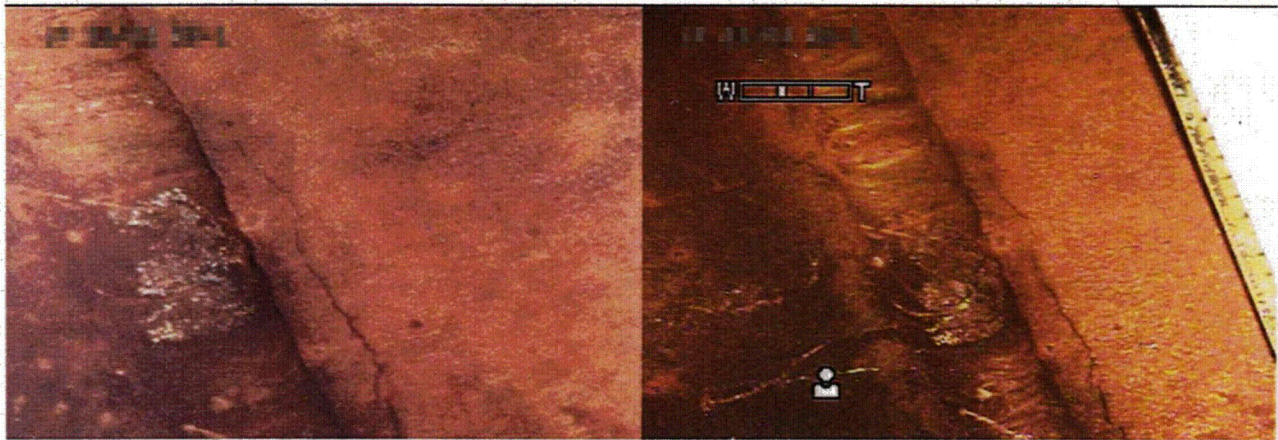
Figure 6.3 A Crack Before (left image) and After (right image) Cleaning Loose Oxide Layer from Surface
