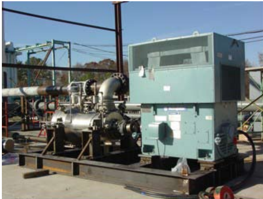
Figure 1– Photograph showing Installation in Test Loop for CA Pump and Motor Test Specimen during facility construction
