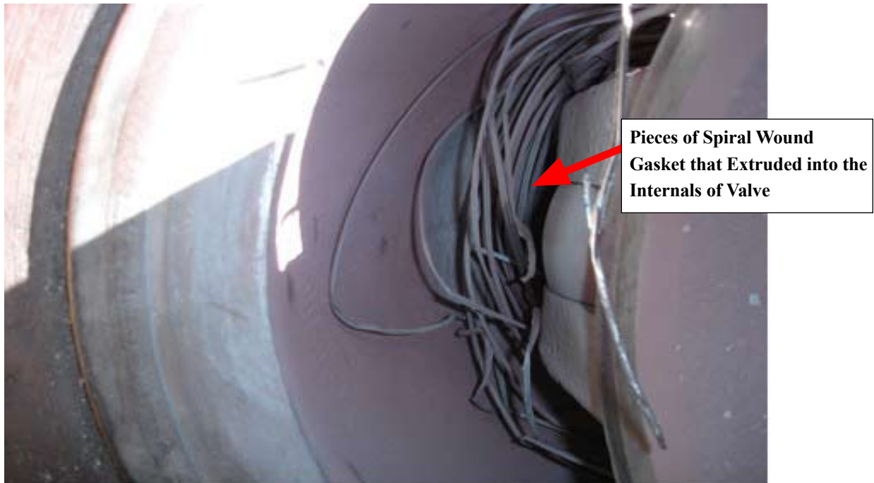
Figure 9 – Internals of a Gate Valve with extruded gasket. Gasket pieces also found in Steam Generator
