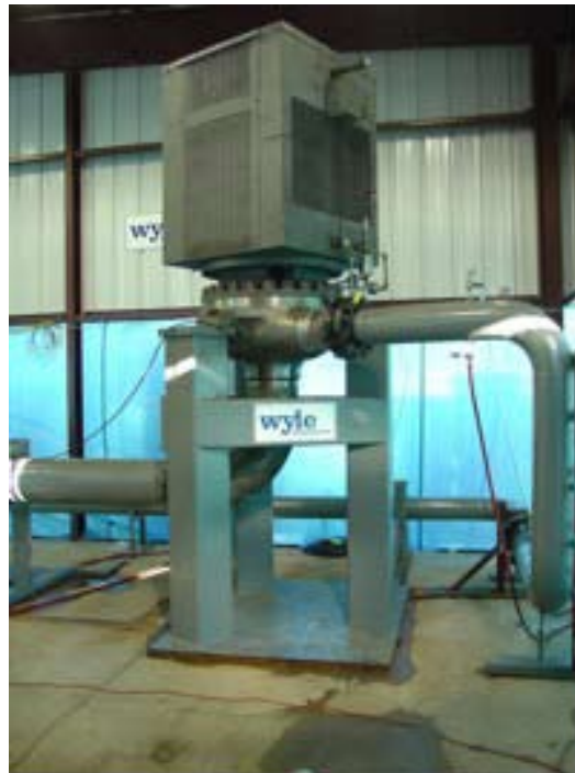
Figure 2 – Photograph showing Installation in Test Loop for WDF Pump and Motor Test Specimen.
