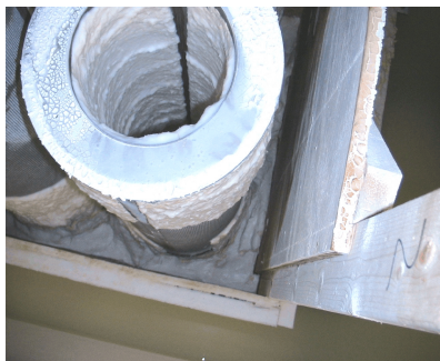
Figure 1 -Strainer in Plywood Enclosure
