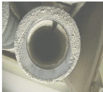
Figure 5 -Debris on top of Strainer
