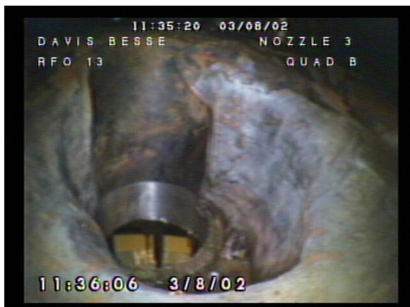
Figure 5 Cavity identified at Davis-Besse during its spring 2002 outage.
