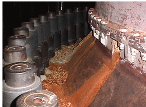
Figure 6 Boric acid and corrosion products identified on the RPV head flange of Davis-Besse during its 2000 outage.
