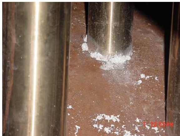
Figure 4 Boric acid deposits identified at Crystal River Unit 3 during its fall 2001 outage.
