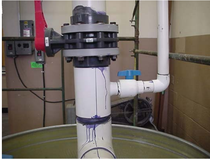
Figure A.10. Intersection of the bases of the 6-in. inner recirculation loop and the 2-in. outer recirculation loop.
