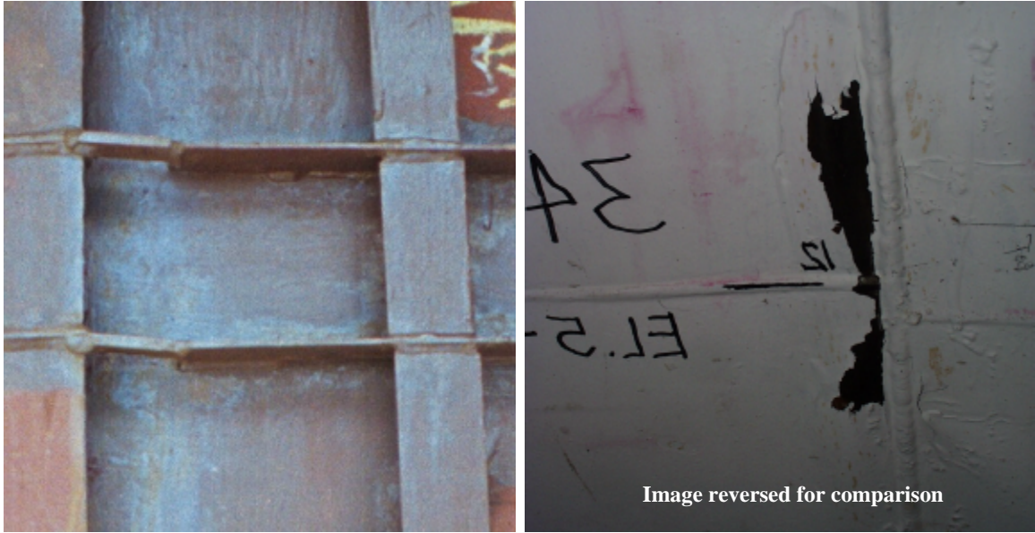
Figure 5.81 Tear #12 at E/H
