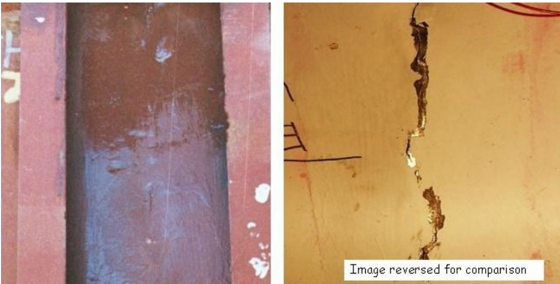
Figure 4. Photographs showing region of tear #4-1 from outside of liner (left) (prior to concrete placement) and inside of liner (right) (prior to removal of paint). Separate tears began of opposite sides of the weld, eventually growing together through the fusion zone.
