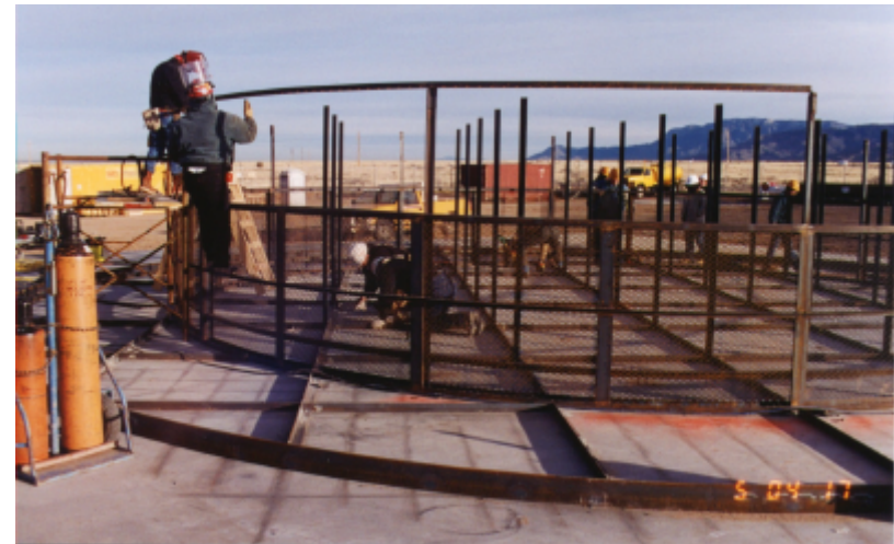
Figure 2.13 Basemat Rebar Support Frame
