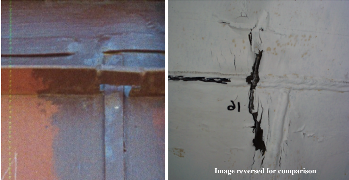
Figure 5.85 Tear #16 at Rathhole Detail
