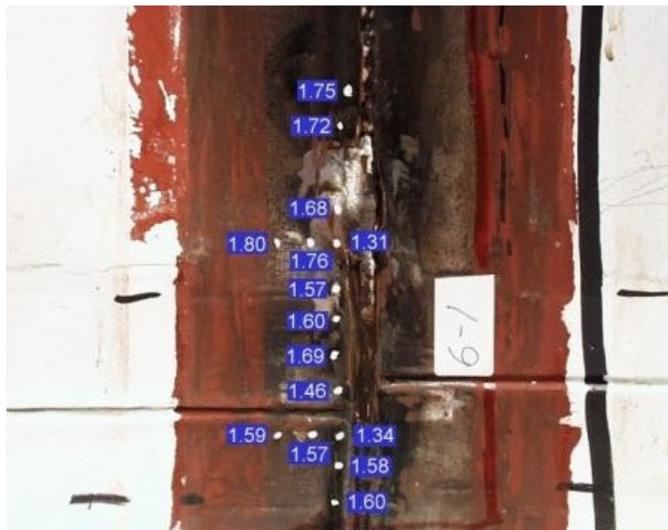
Figure 22. Liner thicknesses (in millimeters) measured ultrasonically in the vicinity of tear #6-1.
