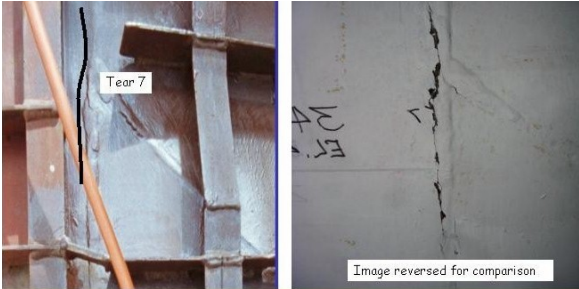
Figure 15. Photographs showing region of tear #7 from outside of liner (left) (prior to concrete placement) and inside of liner (right) (prior to removal of paint).
