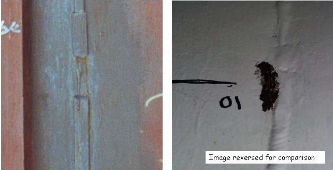
Figure 9. Photographs showing region of tear #10 from outside of liner (left) (prior to concrete placement) and inside of liner (right) (prior to removal of paint). Note missing segment of back-up bar in vicinity of repair weld and tear.
