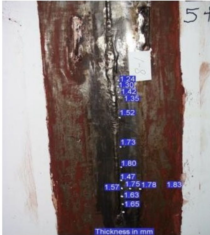
Figure 25. Liner thicknesses (in millimeters) measured ultrasonically in the vicinity of tear #8-1.
