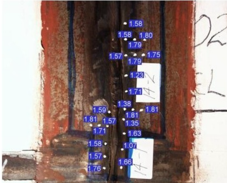
Figure 29. Liner thicknesses (in millimeters) measured ultrasonically in the vicinity of tear #14 (14-1 and 14-2).
