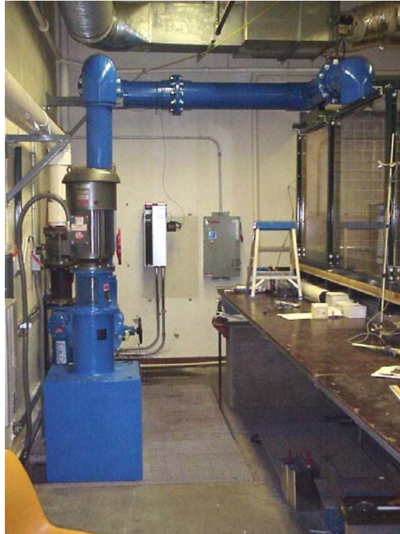
Fig. A-15. Large flume supply pump and overhead piping.
