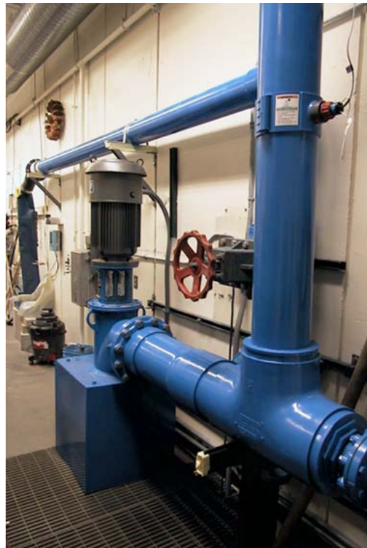
Fig. A-16. Large flume supply pump and in-line flow meter.
