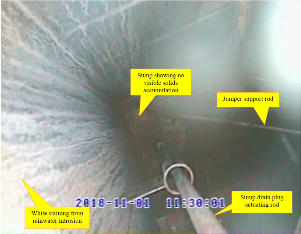
Figure 6. View Looking Down at the FDB-5 Sump (November 2018). Image Credit: Figure 2.4-1 in SRR-CWDA-2020-00011.
