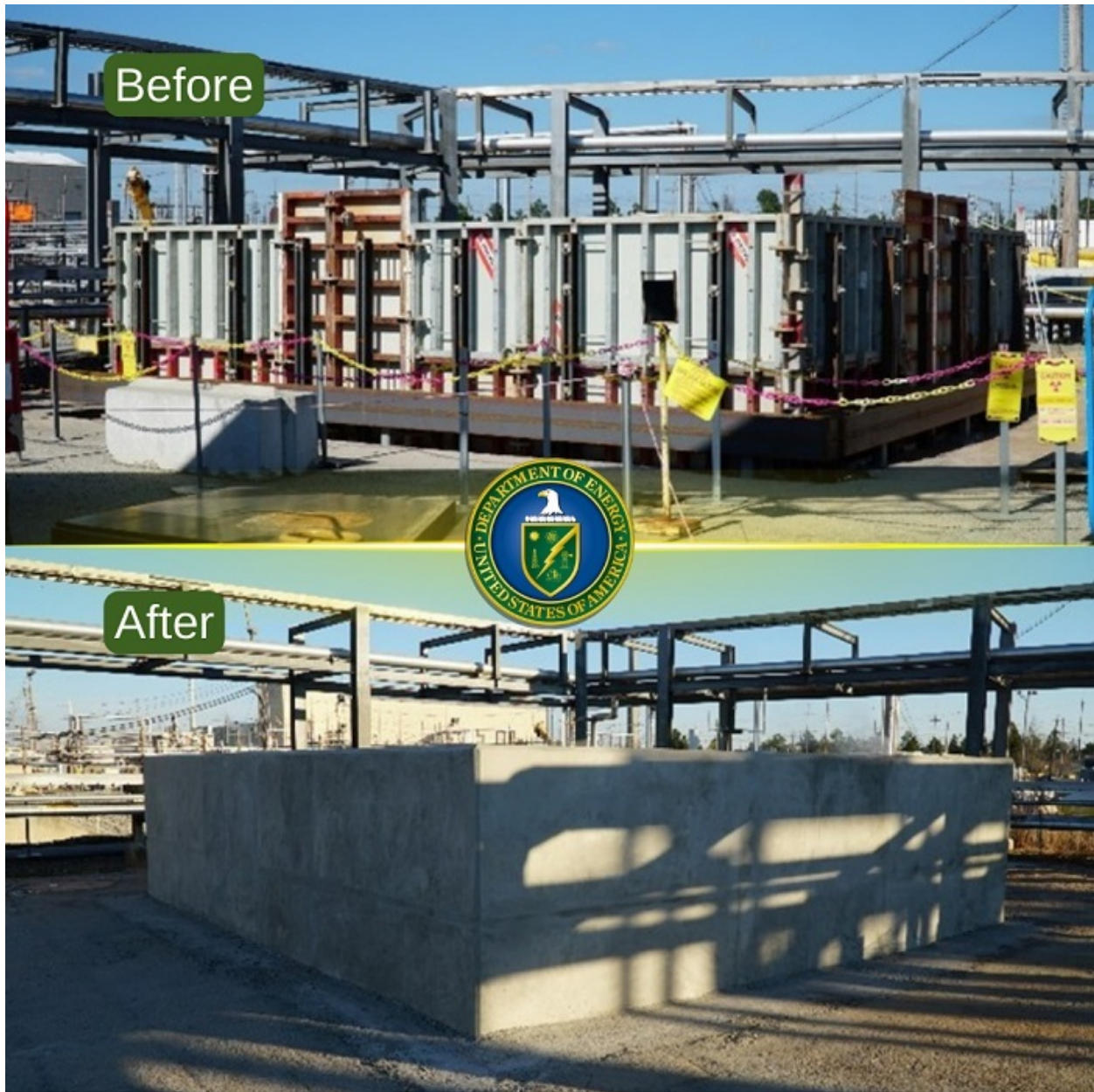
Figure 2. Before (top) and After (bottom) Pictures of FDB-5 Entombment in Concrete. Image credit: J. Beasley “Savannah River Site Grouts, Closes Liquid Waste Structures in Place,” DOE EM newsletter, Vol. 14, Issue 47, December 6, 2022, see https://content.govdelivery.com/accounts/USDOEOEM/bulletins/33abe59 .
