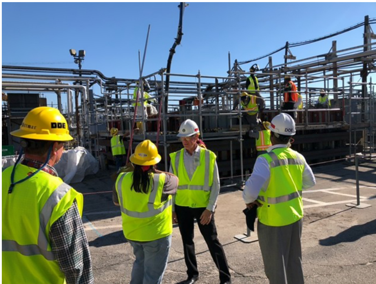
Figure 1 Placement of Concrete Surrounding FDB-6. Image credit: J. Beasley “Savannah River Site Grouts, Closes Liquid Waste Structures in Place,” DOE EM Newsletter, Vol. 14, Issue 47, December 6, 2022, see https://content.govdelivery.com/accounts/USDOEOEM/bulletins/33abe59 .
