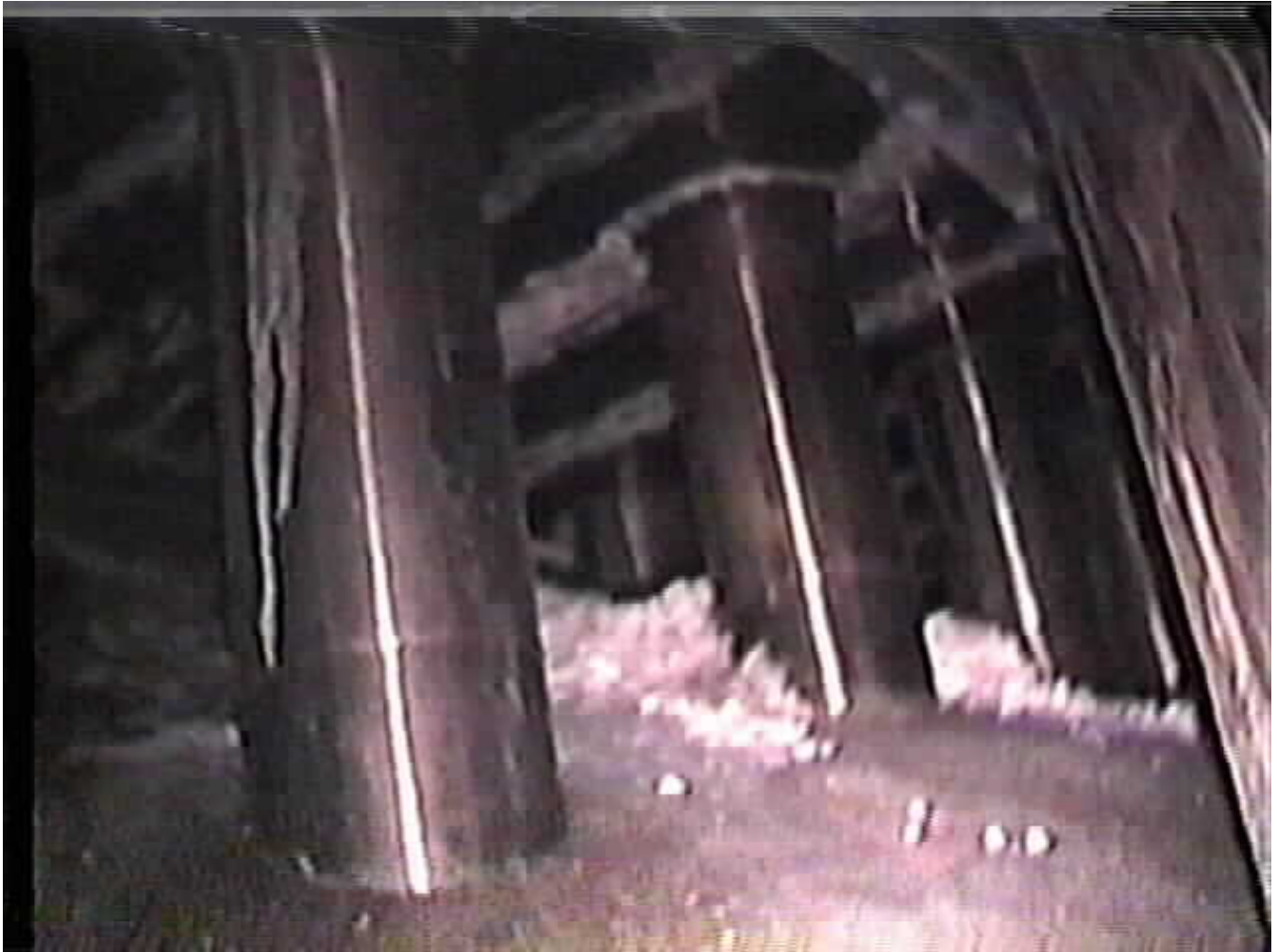
Figure 7.11 Boric Acid Deposits Behind the CRDM Nozzles on the North Side of the Reactor Pressure Vessel Head at 10RFO. 86
