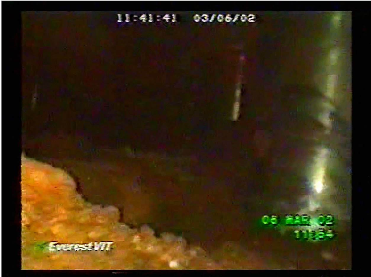
Figure 7.16 Corrosion Product/Boric Acid Deposits Adjacent to Nozzle 3 (270 Degree Side) after Hydrolasing. 106
