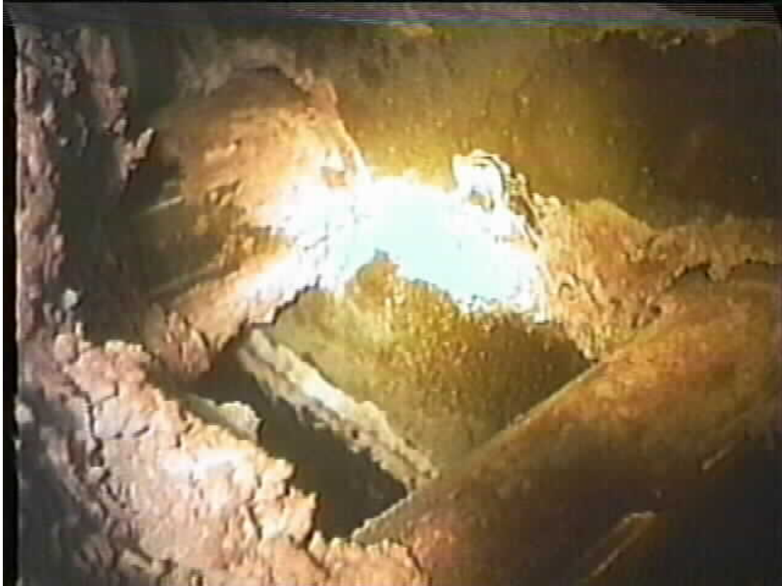
Figure 7.9 Flange Leakage Showing Boric Acid Deposits On Side of Nozzles and Stalactites from Gaps in Insulation (8RFO). 81
