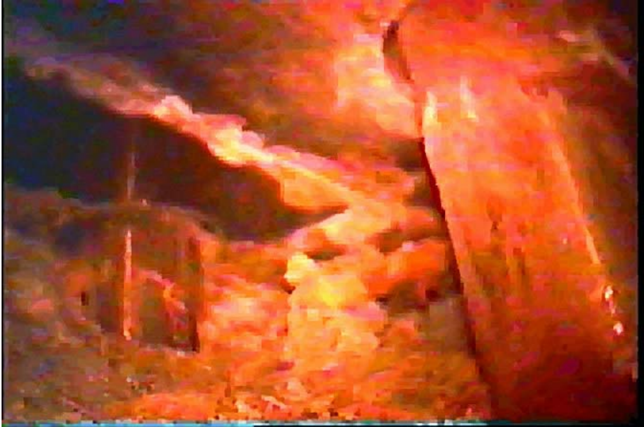
Figure 7.13 Boron Piled Up to the Mirror Insulation Near the Center of the RPV Head (12RFO). 99
