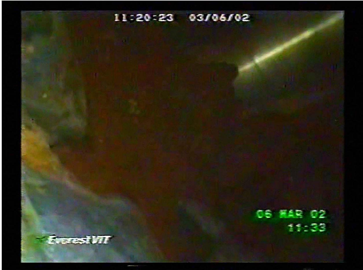
Figure 7.15 Corrosion Product/Boric Acid Deposits Adjacent to Nozzle 3 (90 Degree Side) after Hydrolasing. 105
