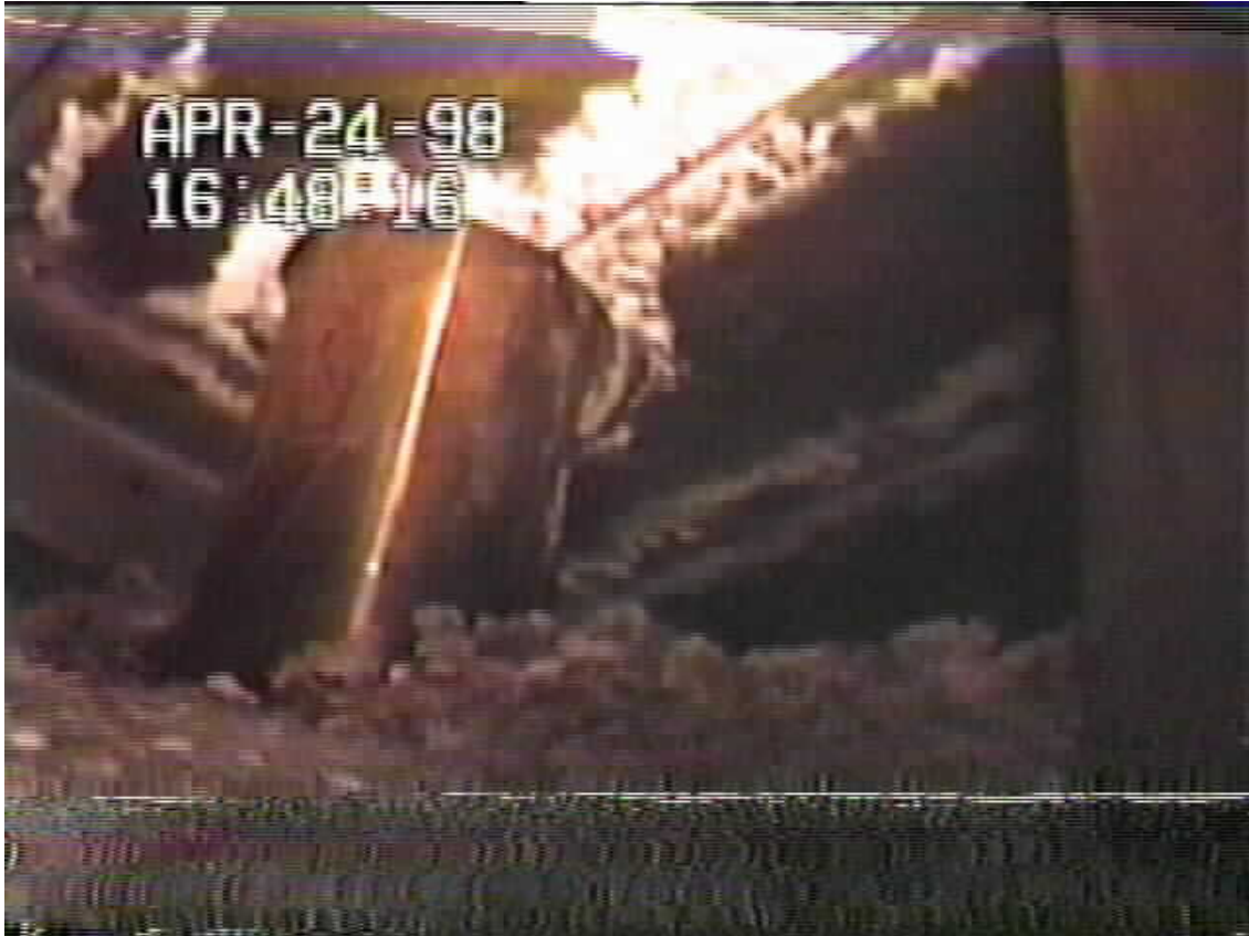
Figure 7.12 Boron Piled on Reactor Pressure Vessel Head Under the Mirror Insulation Near Nozzle 31 (11RFO). 89
