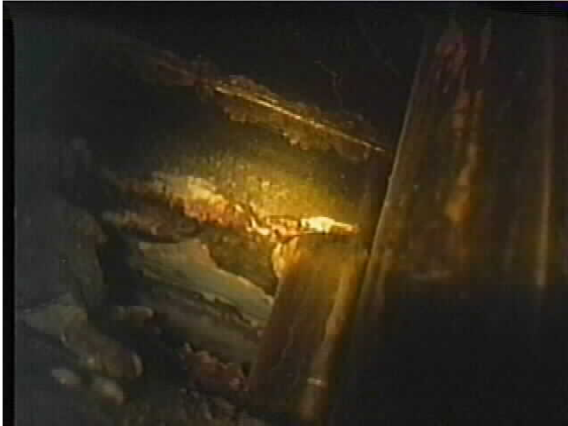
Figure 7.8 Flange Leakage Showing Boric Acid Deposits Leaking Through the Mirror Insulation at 8RFO. 81
