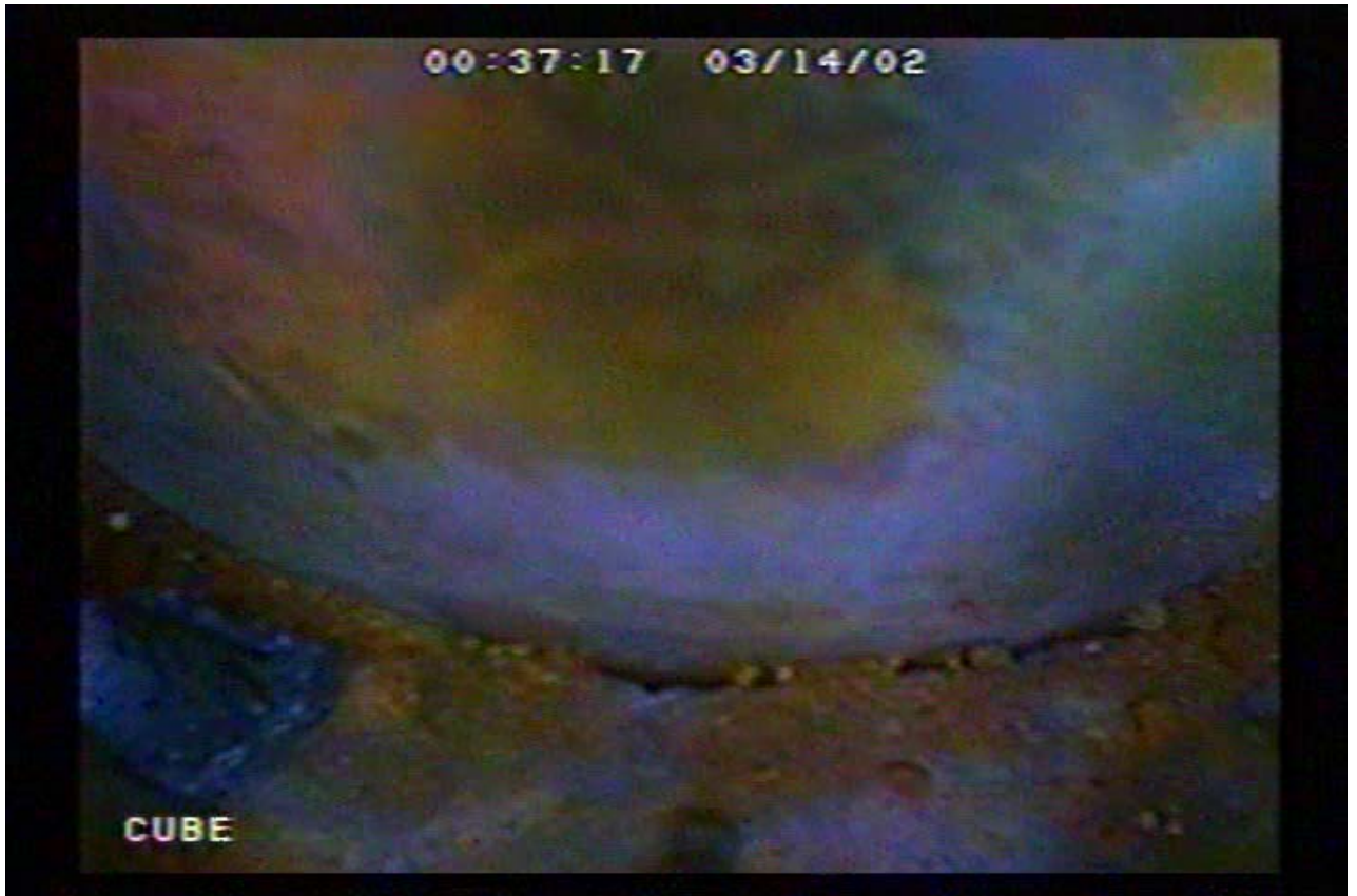
Figure 4.4 Crevice identified by inspection of Nozzle 2 with a hand-held video camera following the removal of a section of mirror insulation. 14
