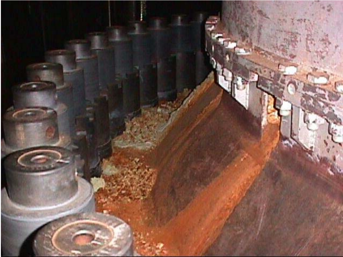
Figure 4.1 Boric acid and iron oxide flowing from mouse holes at 12RFO. 5
