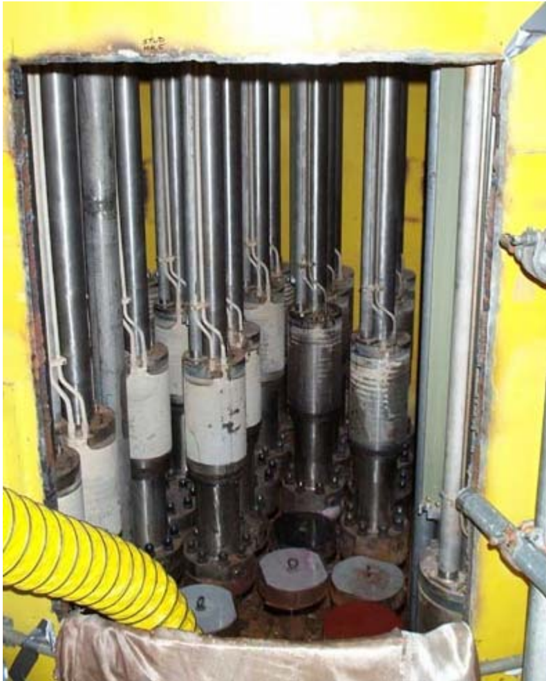
Figure 3.7 View through the Access Opening Cut in the RPV Head Service Structure above the Support Steel and Insulation Showing the Close Proximity of the CRDM Flanges
