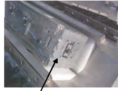
T/N Close-up: No Significant Damage to Top head or Moderator Blocks.
